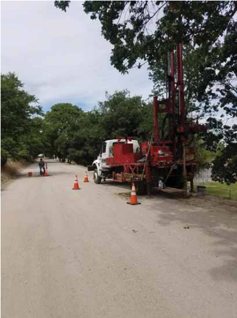
Performing infiltration test to determine permeability of existing soil in bore hole (left) and preparing to drill another hole (right)
