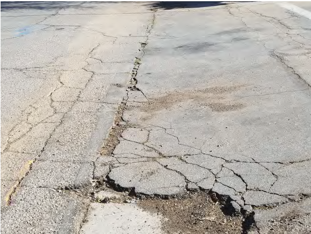
Deteriorated pavement due to the lack of adequate drainage improvements.
