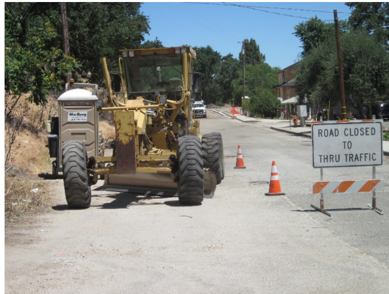
Construction has begun to pave the dirt area of Vine Street, behind Georgia Brown Elementary School (06/21/2018)
